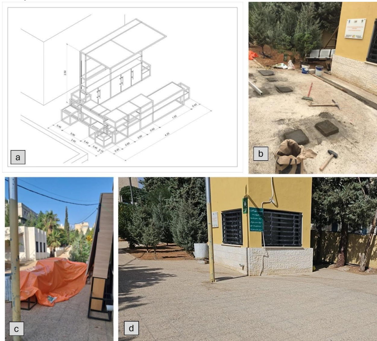
Figure 3. a: The Project 3d model, b: Preparing the site for implementing the project, c: Transfer the project on-site, d: The Project site in the Queen Noor Park.
